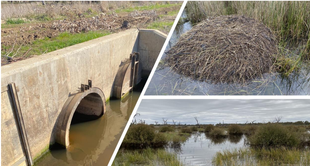
Figure 9: Vandalism of regulator at Gaynor Swamp and the effects to the swamp from this.
