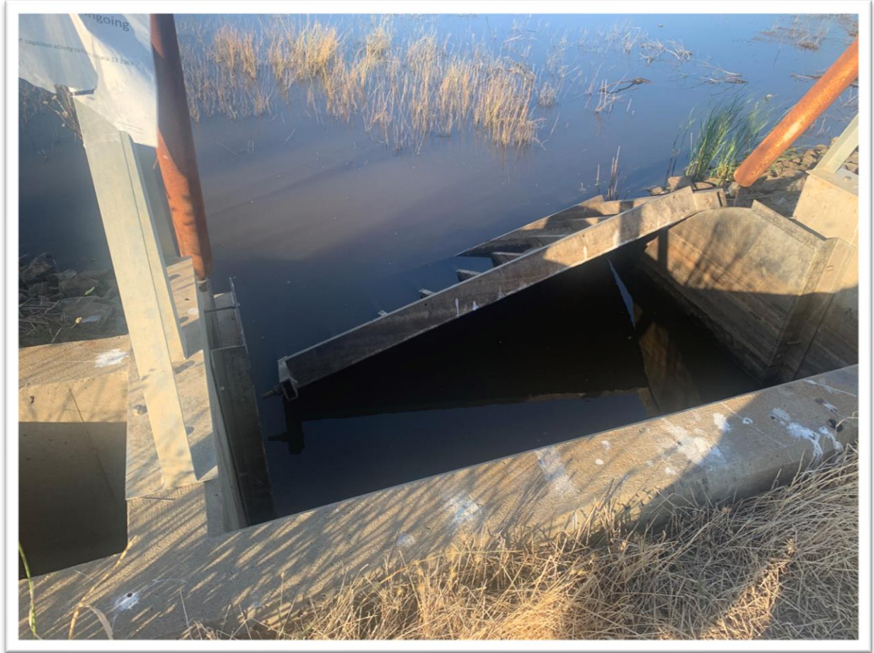
Figure 6: Damage to the regulating structure at Gaynor Swamp due to vandalism in October 2022.
